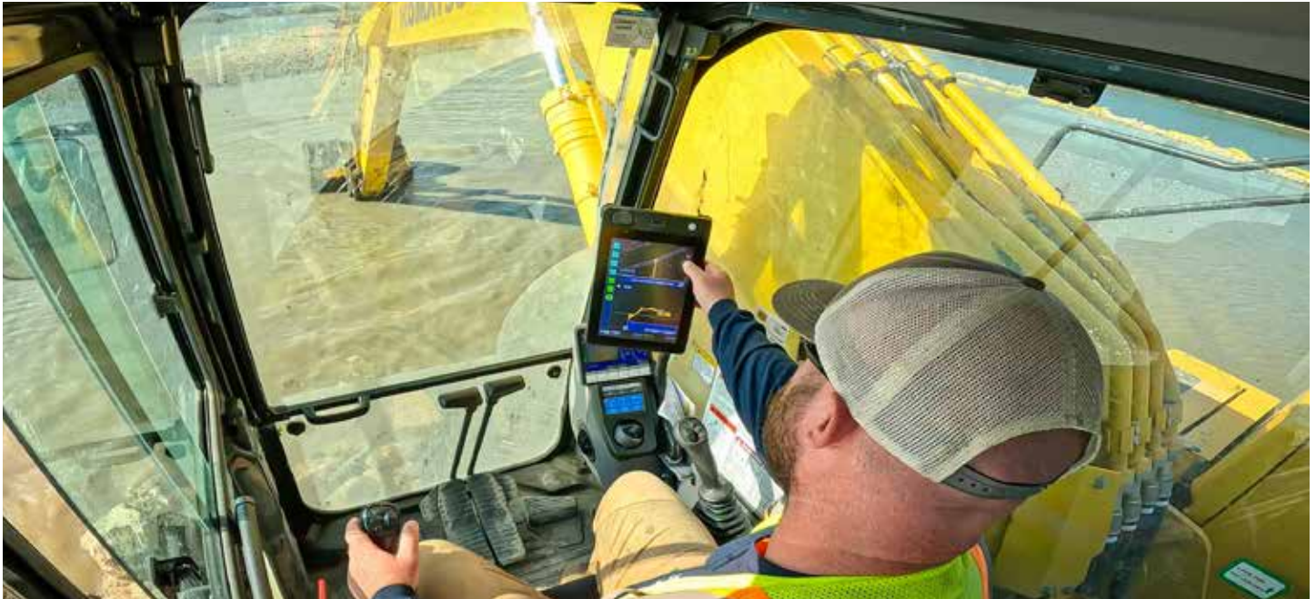
Komatsu PC210LCi operator Ryan McClure confirms settings while working on Clark Island. Restoration work will allow the Maumee River Islands to capture sediment, reduce erosion and improve wildlife habitats and ecological systems.
