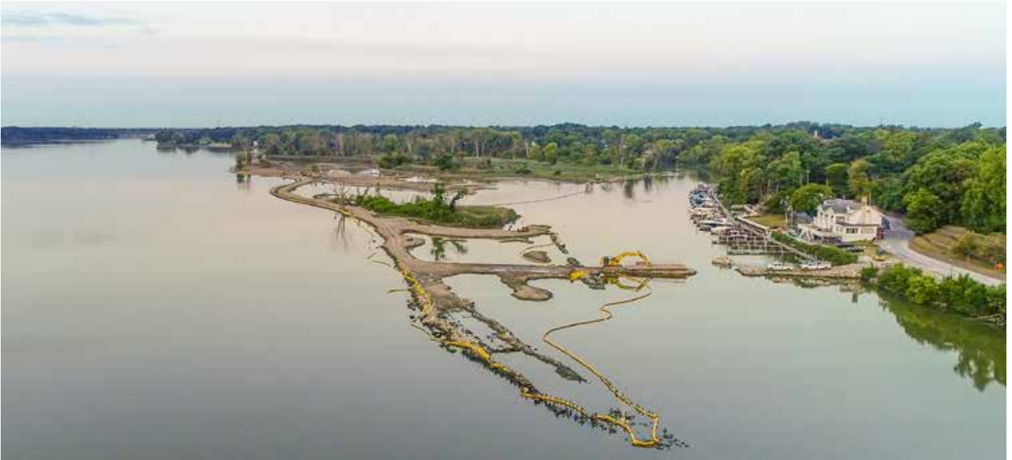
Pictured: Horseshoe Delaware and Delaware (foreground) portions of the project. The use of Komatsu iMC equipment and GPS technology allowed the company to increase capabilities, accelerate project completion by 6-7 months and improve safety.
