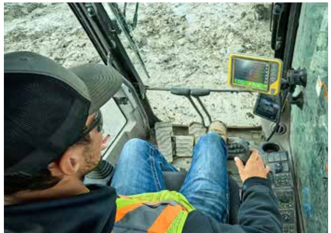
Topcon technology allows Operator Tony Gregory and an amphibious pontoon excavator “to make the impossible possible.”
