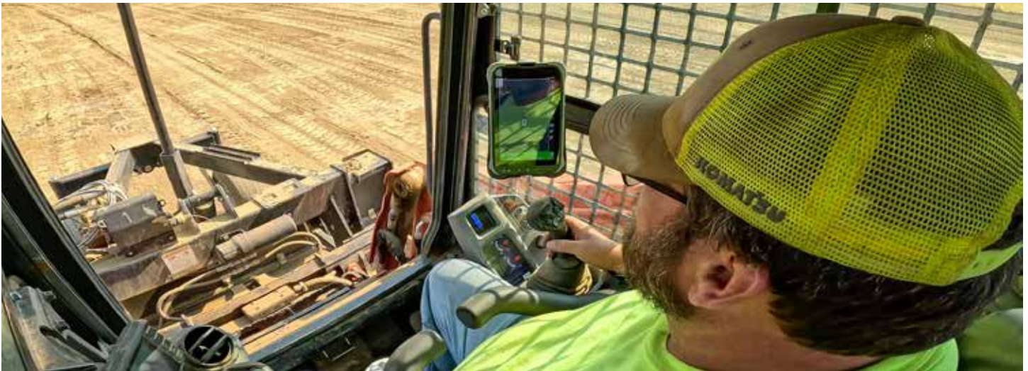
Operators are rarely excited about learning new systems. That said, Environmental Trenching Inc.'s Operator John Shafer (above) and crew were all-in on Topcon's MC Mobile System once they saw how easy it was to use.
