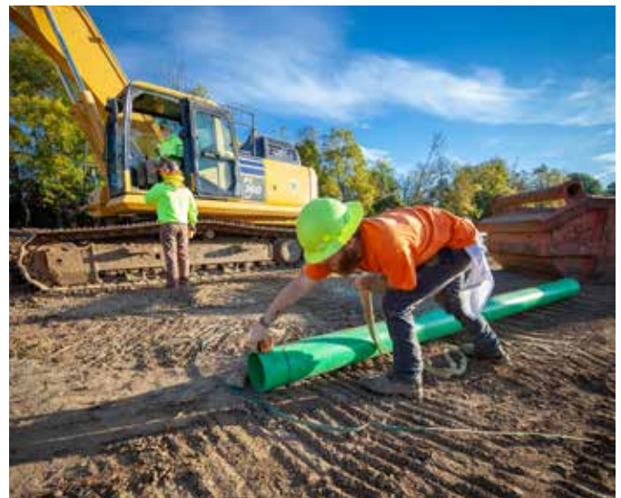
MDX Inc. vice president Eric Dedden (rear left) discusses operations on a Franklin, Ohio site with Operator Mike Dedden as Pipelayer Tylor Griffin prepares pipe.
