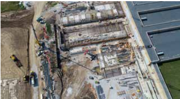
With a working radius of 190 feet, the 110-ton Link-Belt 218 HSL commands access to the entire, active work zone at the company's $55-million Collins Park Water Treatment Plant Basins 7 & 8 Project.
