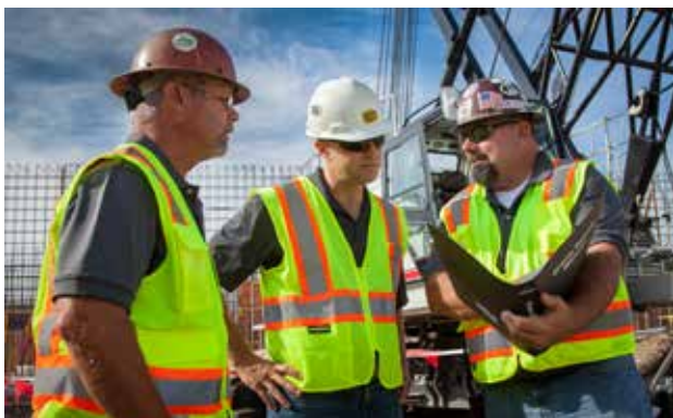
Mosser Construction operators Mark Rosenberger (left) and Chris Smith (right) discuss the Link-Belt 218 HSL's load capacity chart with Columbus Equipment Company's Luke Matheson.
